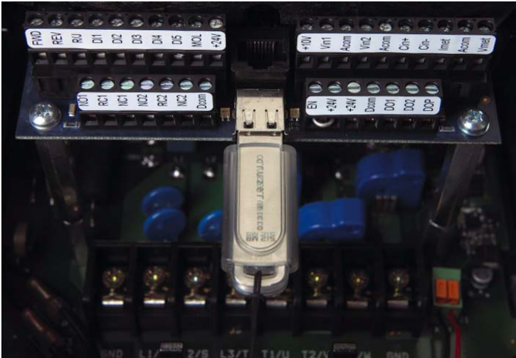
Figure 9: Vacon 500x Control Terminals
